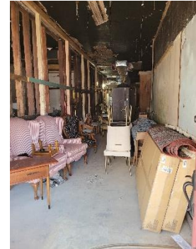
Valuable and fragile items had to be carefully moved for demolition to begin.
